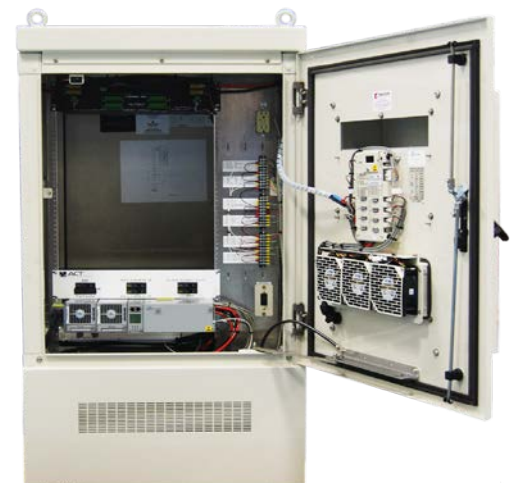
Mobile Backhaul Base Cabinet
